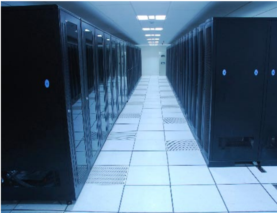
The Siemens PLM Software Centre 10G Data Centre in Pune: Future Ready with AMP NETCONNECT Cabling Solutions
