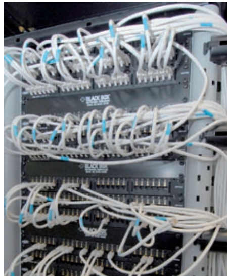
The AMPTRAC patch panels enable the patch status of each individual port to be traced.
